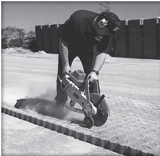
Figure 8-15: Wheeled dry saw increases speed and accuracy for paver cutting. However, they wear out saw blades faster and require great attention to safety during cutting.
